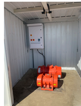
One of four sets of SOVs installed near the RTE plant.
